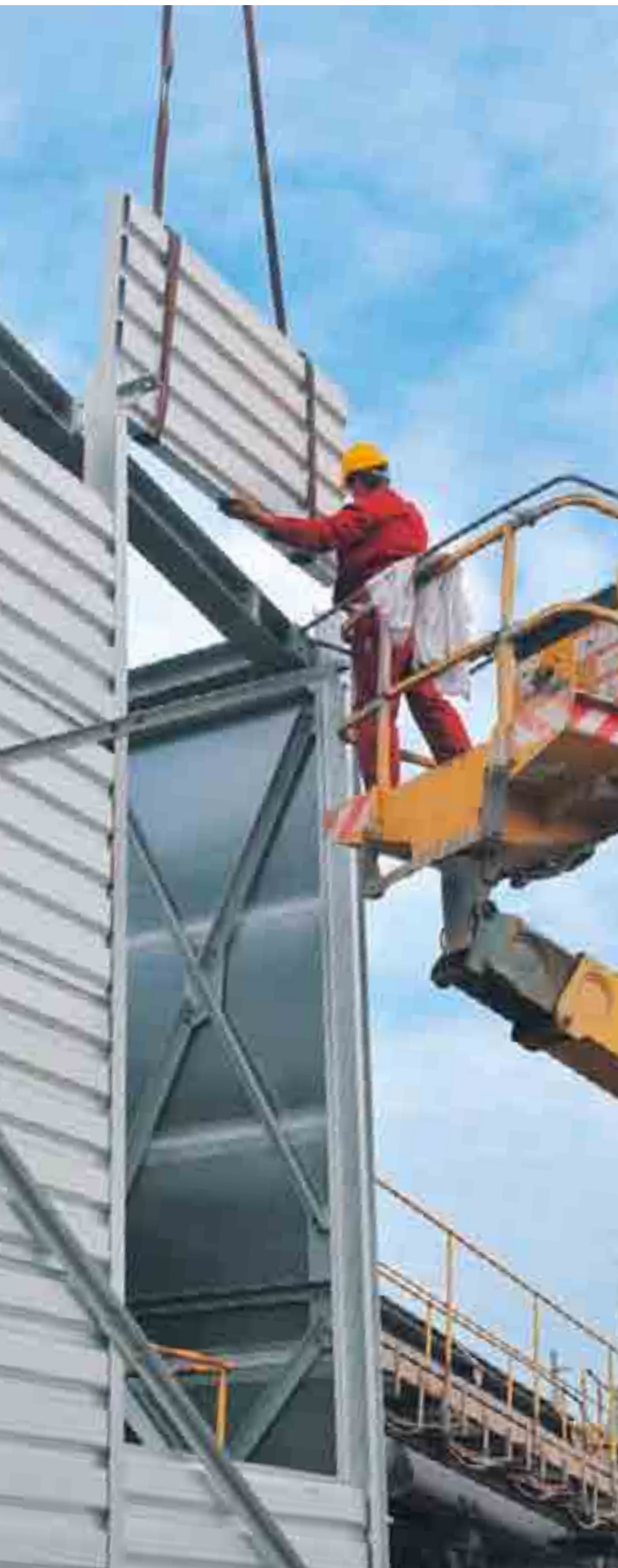
Sound insulation cover of an actuator station at the lignite opencast pit in Schleenhain
