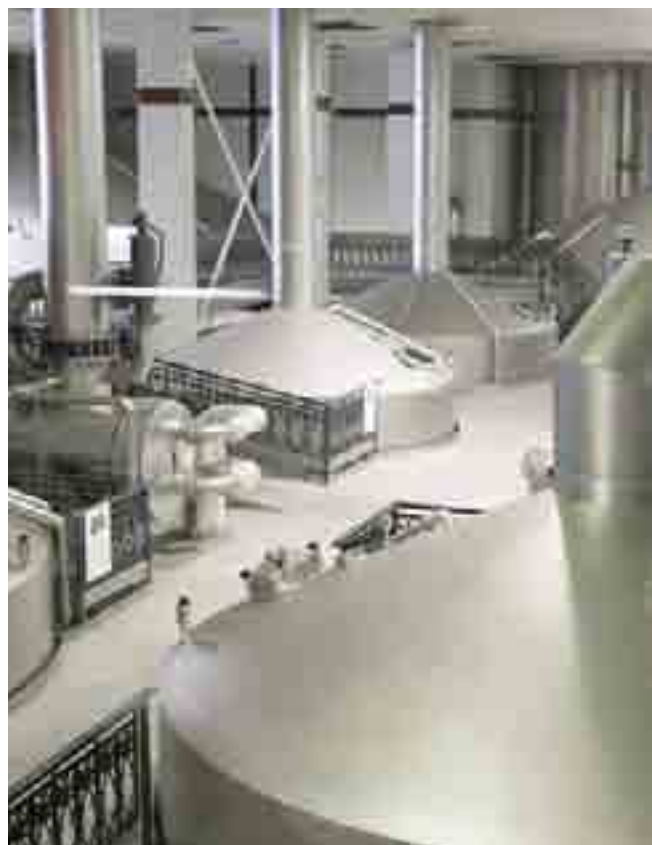
Hygienic, flawless insulation in a brewery in Bavaria
